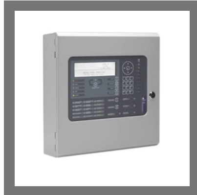
Fire Security Alarm Control Panel
