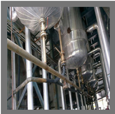
Multiple Effect Evaporation System
