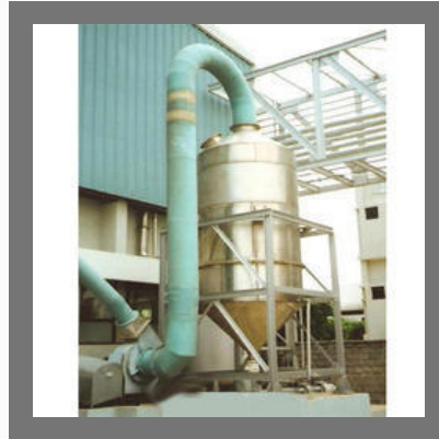
Packed Bed Scrubber
