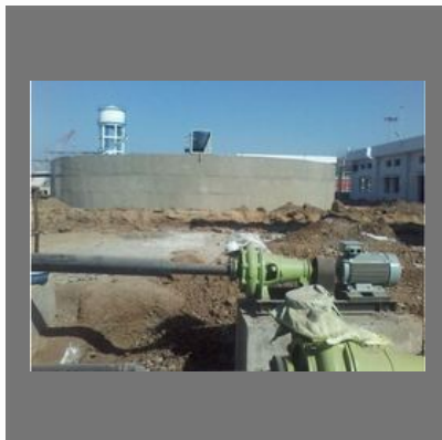
Waste Water Treatment Solutions
