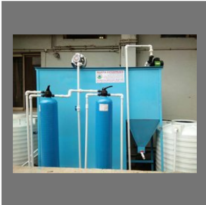
Operation & Maintenance Of ETP
