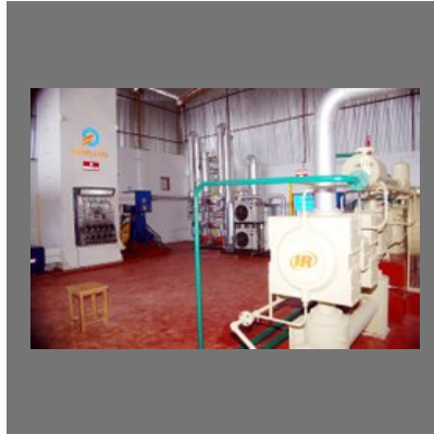
Liquid Oxygen Nitrogen Plant
