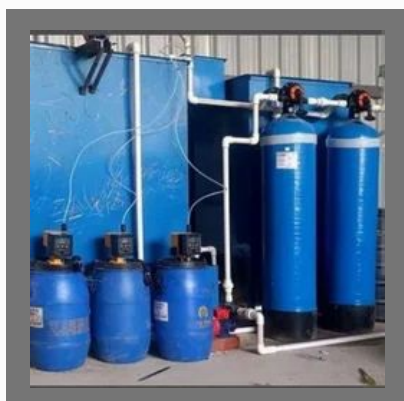
Stp Operation Maintenance Service
