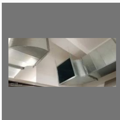
Kitchen Duct Cleaning Services
