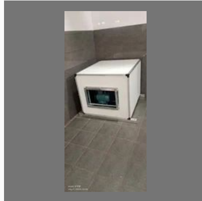
Ahu Installation And Services
