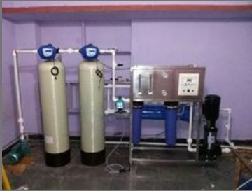
Reverse Osmosis Plant
