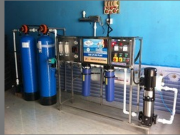
Commercial Reverse Osmosis Plant
