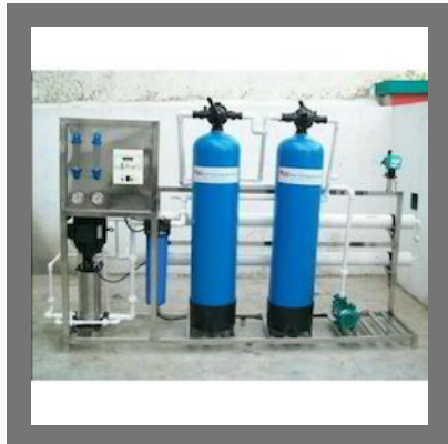
Commercial RO Plant
