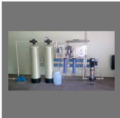
Domestic RO Plant
