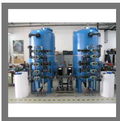
Iron Removal Filter
