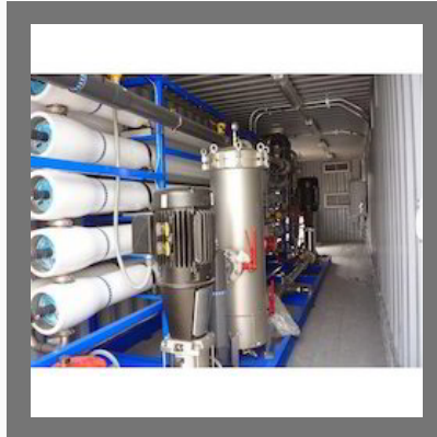
Reverse Osmosis Water Treatment Plant
