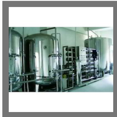
RO Water Treatment Plant
