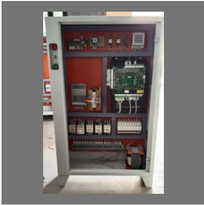
Close Loop Control Panel
