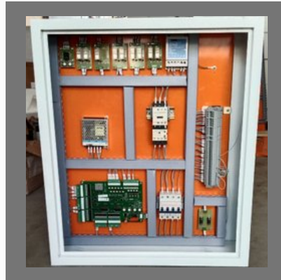
Hydraulic Control Panel
