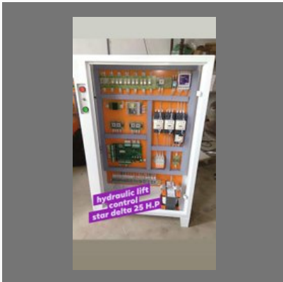
Hydraulic Lift Control Panel
