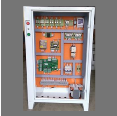
Hydraulic Control Panel
