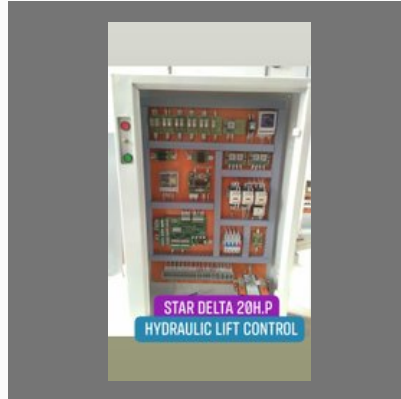
Hydraulic Lift Control Panel
