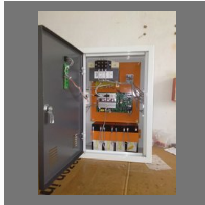
Hydraulic Control Panel
