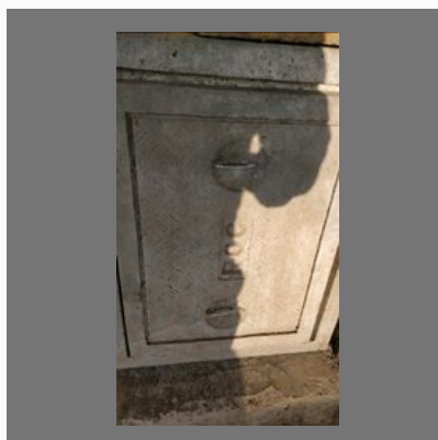
Cement Manhole Cover
