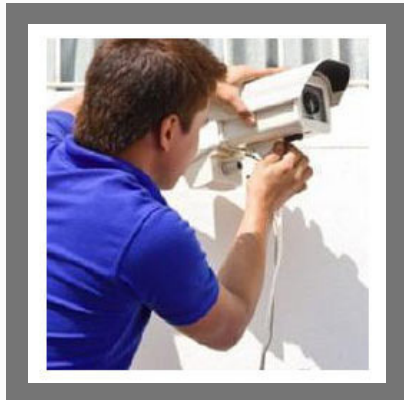
CCTV Camera Maintenance Service
