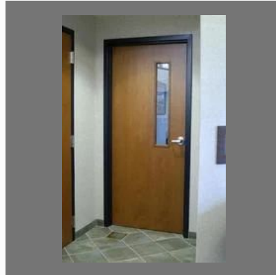
Fire Door With Vision Panel
