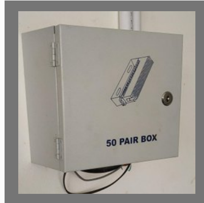
50 Pair Solar Panel cabinet Box
