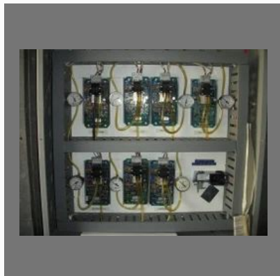
DDC Control Panel
