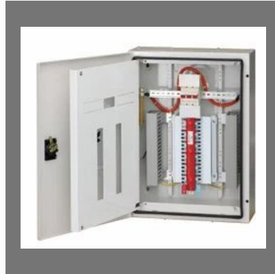
Distribution Panel Board
