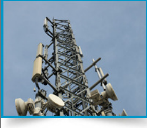
B.T.S Installation, Commissioning & Integration.
