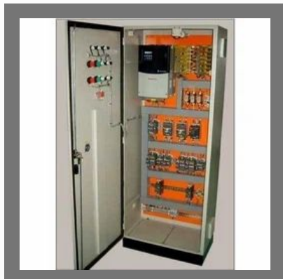
Electric Control Panel
