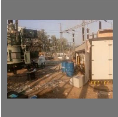
Dehydration & Filtration Of Transformer Oil Services Work
