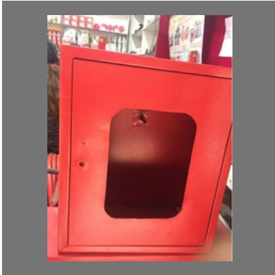
Fire Hose Box
