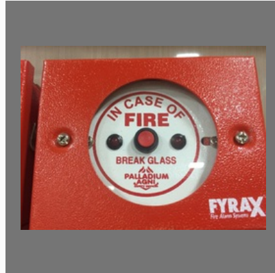
Security Fire Alarm
