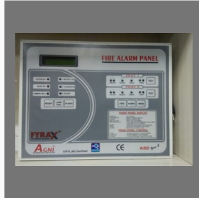
Fire Alarm Control Panel
