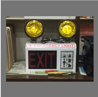
Emergency Exit Lights
