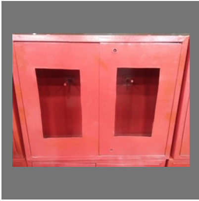
Fire Hose Box
