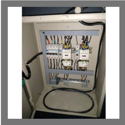
Electric Circuit Panel
