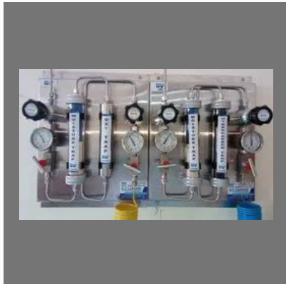
gas purification panel
