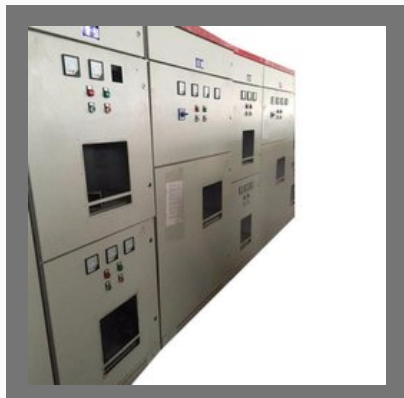
Main LT Control Panel
