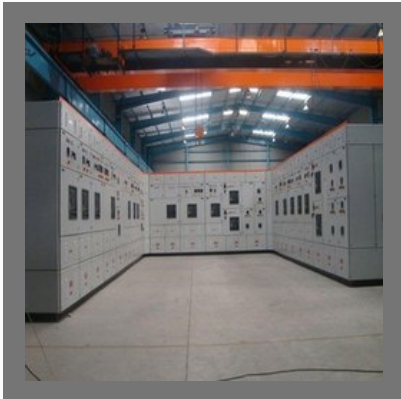
LT Electric Control Panel
