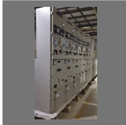
12 KV HT Panel
