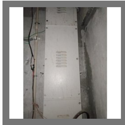
Rising Mains Electrical Box
