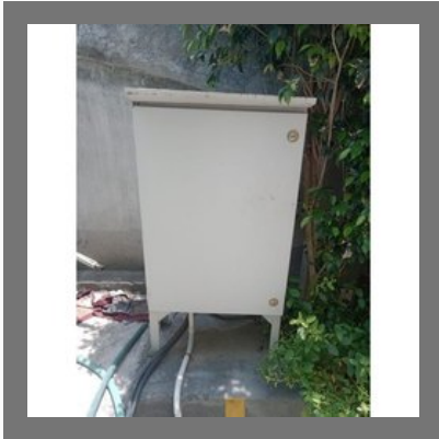
Street Light Control Panel
