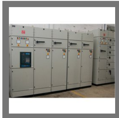
Three Phase APFC Panel
