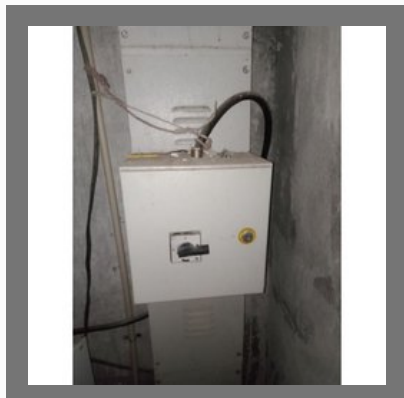
Tap Off Electrical Box
