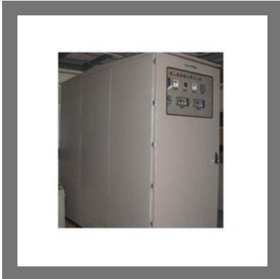
33 KV Outdoor HT Panel
