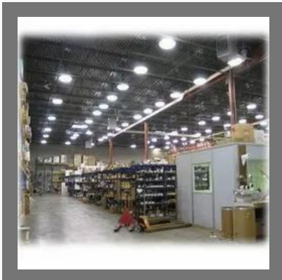
Industrial Lighting Service
