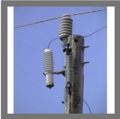
Lighting Arrester Services
