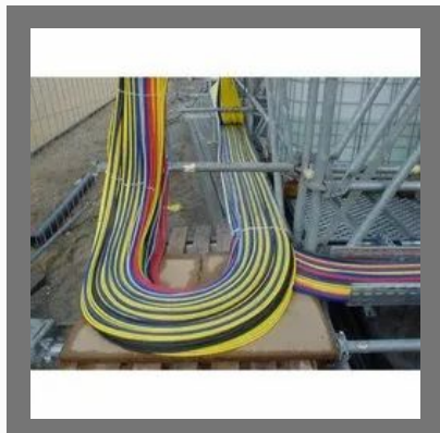
LT Installation Service
