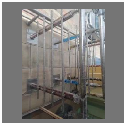
Stainless Steel Pipes
