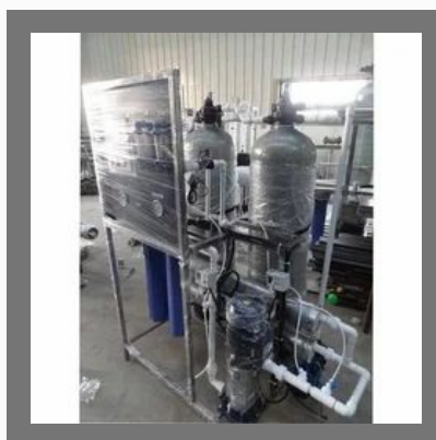
Reverse Osmosis System
