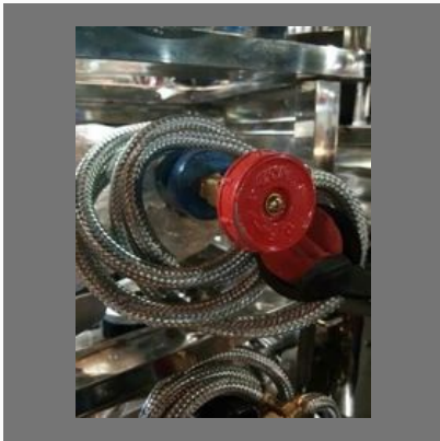
Gas Stove Pipes
