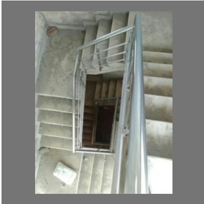
Stainless Steel Stairs Railing
