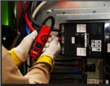
Electrical And Automation
