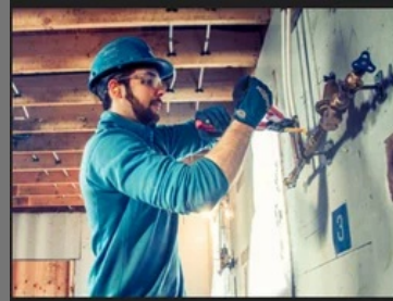
Plumbing And Piping
