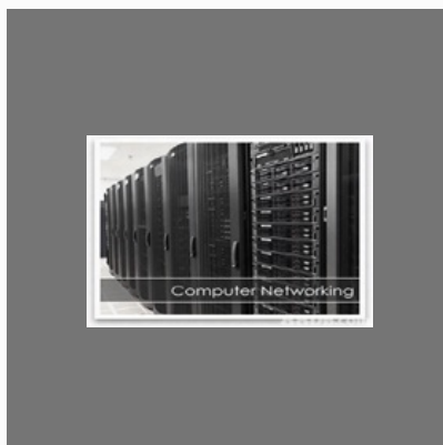
Server & Switch Racks
