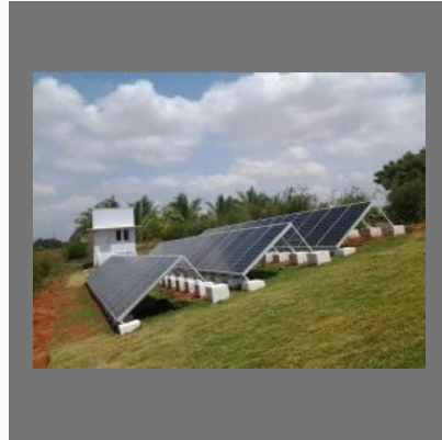
Solar Water Pumping Systems
