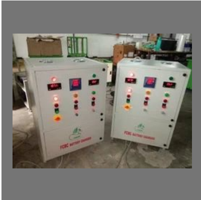
Substation Battery Charger
