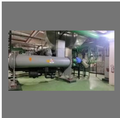
Pawoi Plant Room
