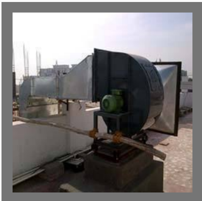
Industrial Ducting Service
