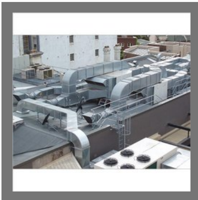
Industrial Ducting Service
