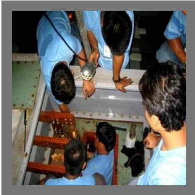
Voltage Stabilizer Transformer Installation Services
