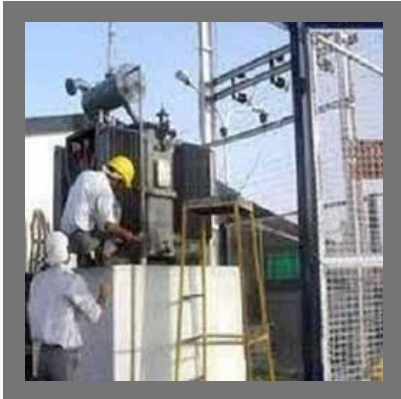
Auto Transformer Maintenance Service
