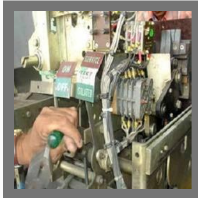
Power Distribution Transformer Maintenance Service
