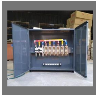
Lt Distribution Box 200 Kva Double circuit
