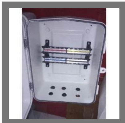
SMC Distribution Box
