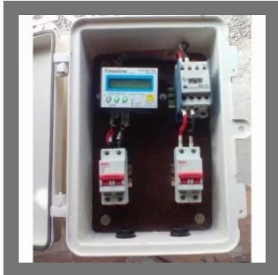
Street Light Timmer Control Panel
