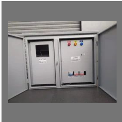
CCMS Street Light Control Panel single phase
