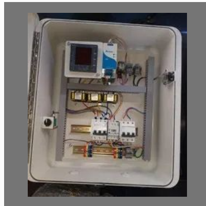
IOT Based Control Panel
