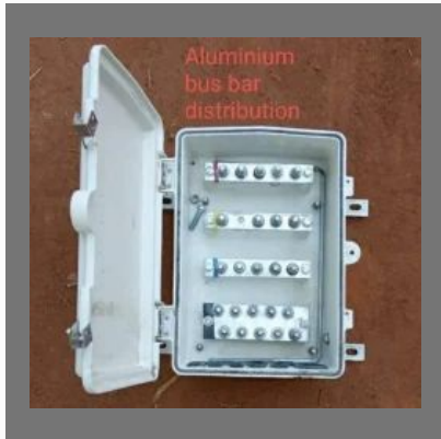
Smc Distribution Box
