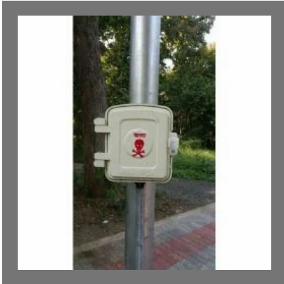
Street Light Pole Box
