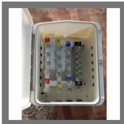
Three Phase SMC Distribution Box
