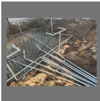
Swimming Pool Plumbing Service
