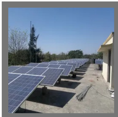
Solar Power Systems
