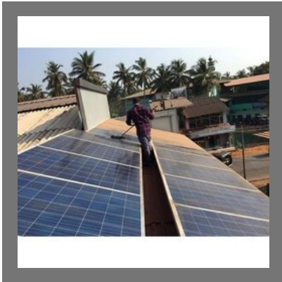
5kW On grid Solar Power Plant
