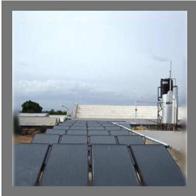
10 kW On Grid Solar Panel System
