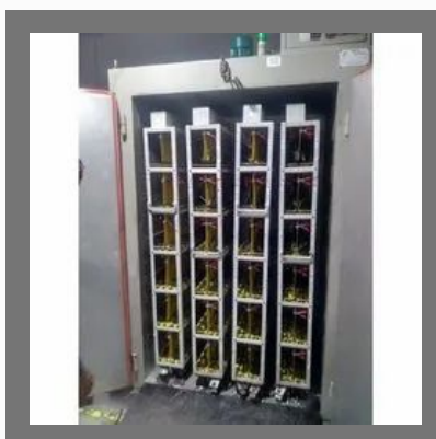
Panel Board Fabrication Service
