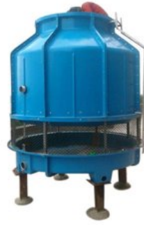
FRP Cooling Tower
