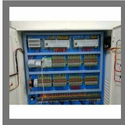
Electric Control Panel
