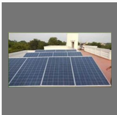
Domestic Solar Power Plant
