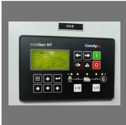
Dg Generator Control Display
