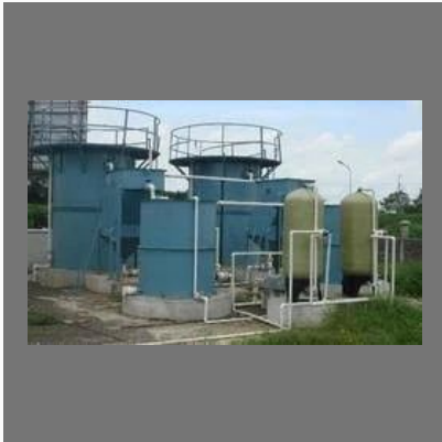
Sewage Treatment Plant
