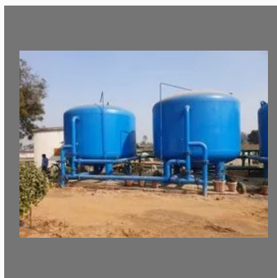
Industrial Water Treatment Plant
