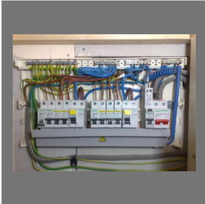
Electrical Distribution Panel Box
