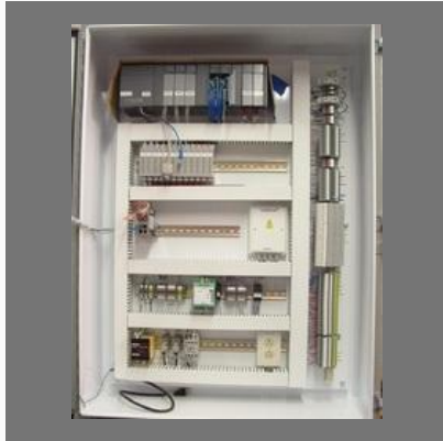
PLC Automation Control Panel
