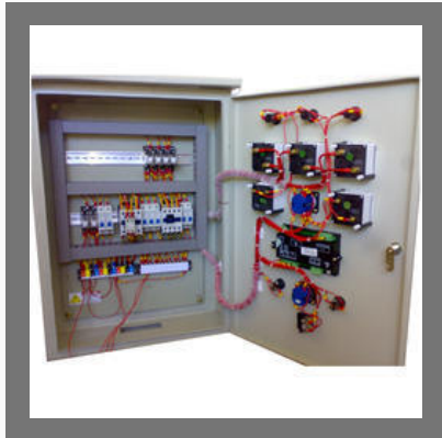
Synchronized AMF Panel
