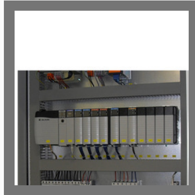
PLC Based Control Panel
