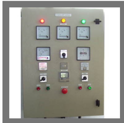
Small MCC Panel
