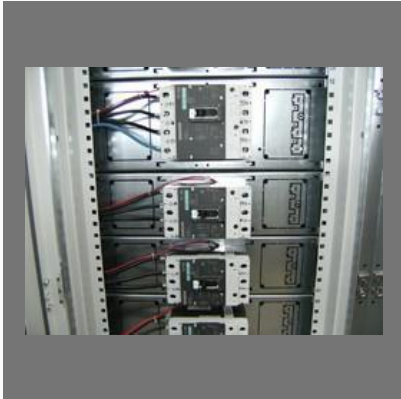
Electrical Distribution System
