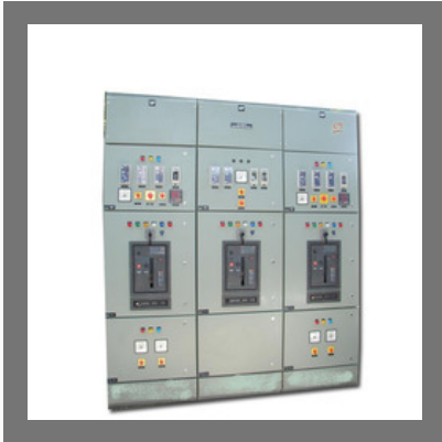
DG Set Control Panel
