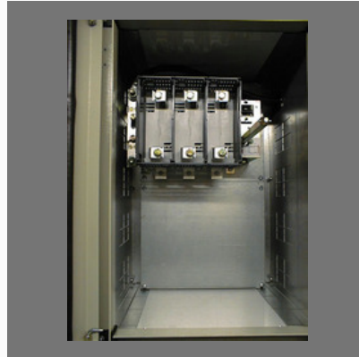
Residential Electrical Distribution System
