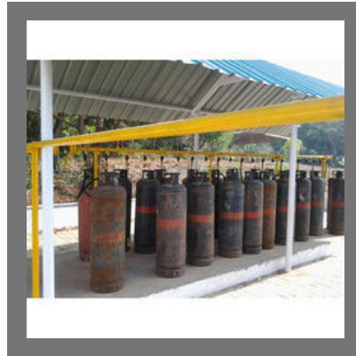
LPG Gas Pipeline
