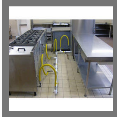
Commercial Kitchen Gas Pipeline
