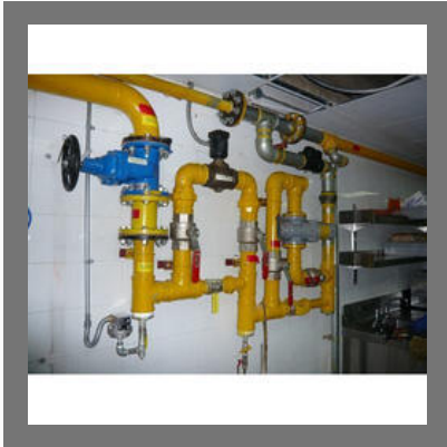
Commercial Gas Pipeline
