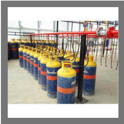
Industrial Gas Pipeline
