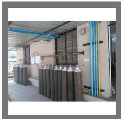
Medical Gas Pipeline
