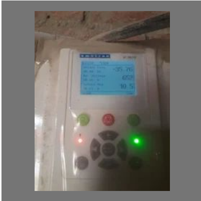
Solar Vfd Drive
