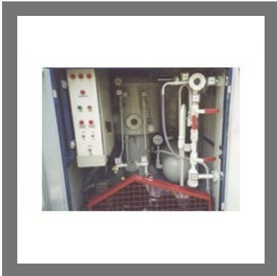
Insulating Oil Conditioning Plant
