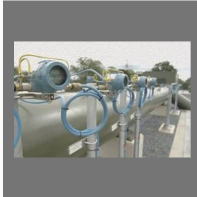
Electrical & Instrument Engineering
