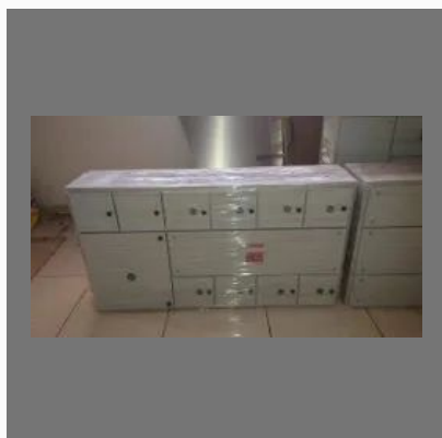
Control Panel Board
