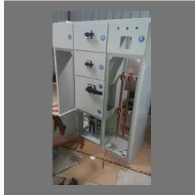
Control Panel Board
