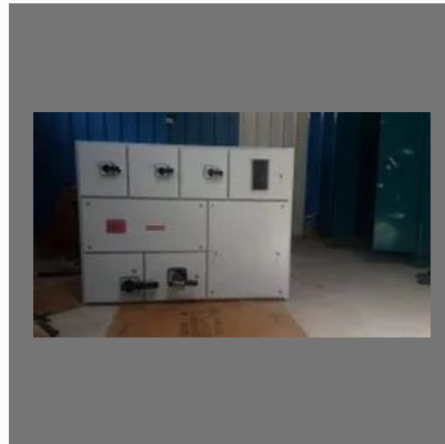
Control Panel Board
