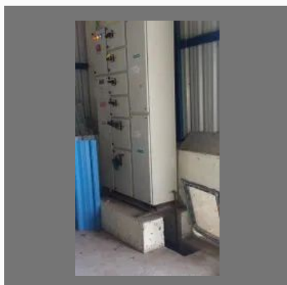
Control Panel Board
