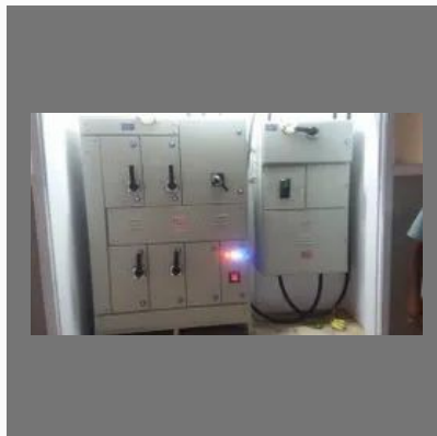
Control Panel Board
