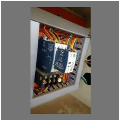
Control Panel Board
