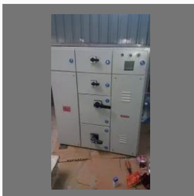
Control Panel Board
