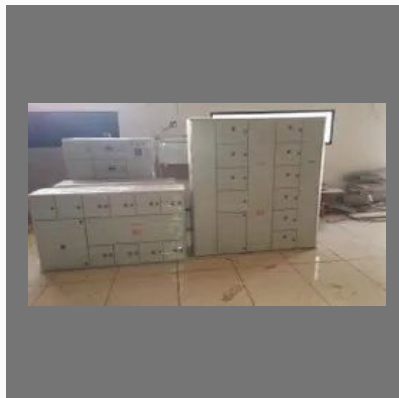
Control Panel Board
