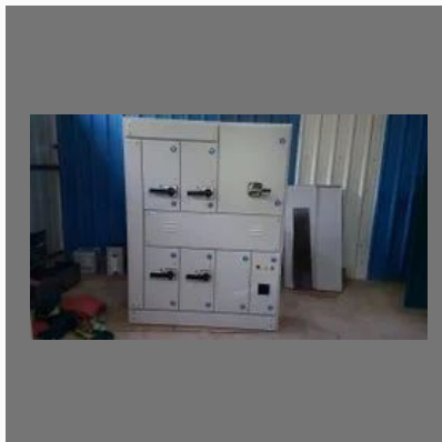
Control Panel Board
