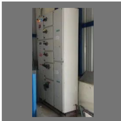
Control Panel Board
