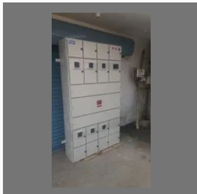
Control Panel Board
