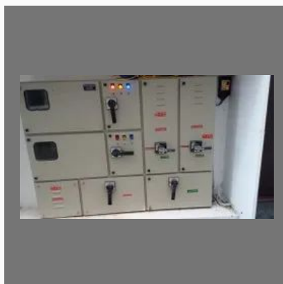
Control Panel Board
