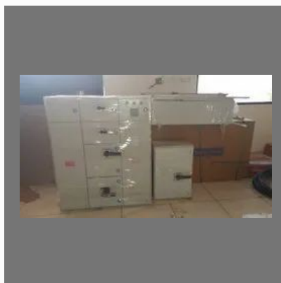
Control Panel Board
