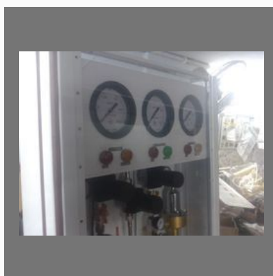
Medical Gas Meter
