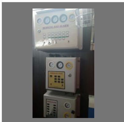
Medical Gas Alarm Panel
