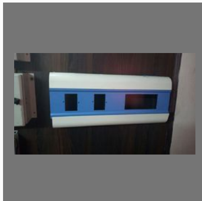
Medical Gas Switch Board
