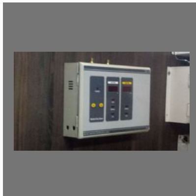
Gas Control Panel
