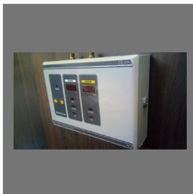
Gas Control Panel
