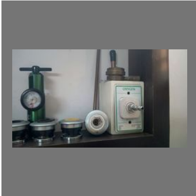
Medical Gas Equipment
