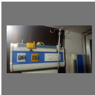
Medical Gas Control Board
