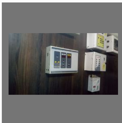
Medical Gas Control Panel
