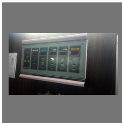
Gas Meter Control System
