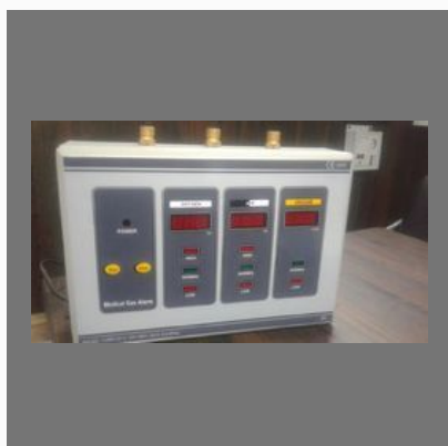
Gas Control Panel
