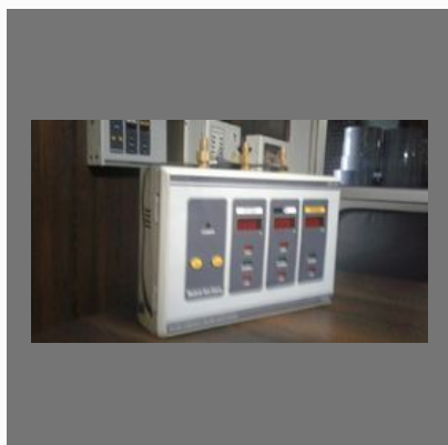
Gas Control Panel
