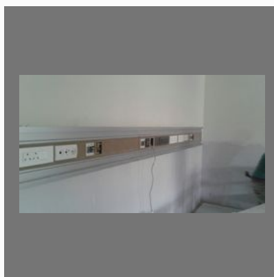
Electronic Long Switchboard
