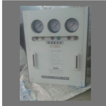
Oxygen Automatic Control Panel
