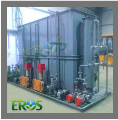
Sewage Treatment Plant (STP)
