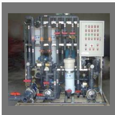
Automobile Effluent Water Treatment Plant
