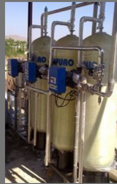
Water Softening Plant
