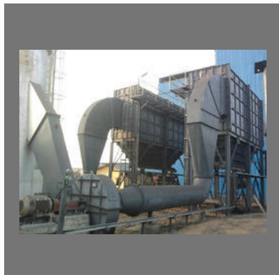
Air Pollution Control System
