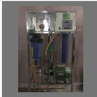
Compact Reverse Osmosis unit
