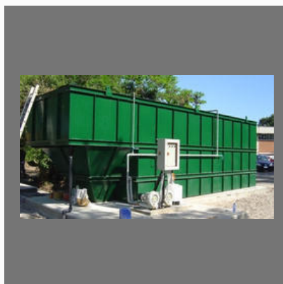
Sewage Treatment Plant ( House, Apartments, Industrial)
