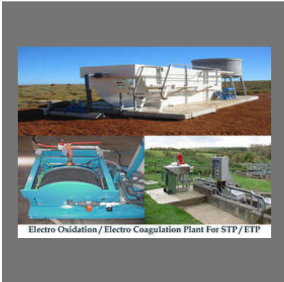
Electro Coagulation Sewage Treatment Plant
