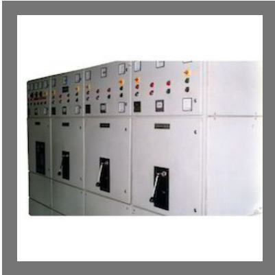
Power Control Panel
