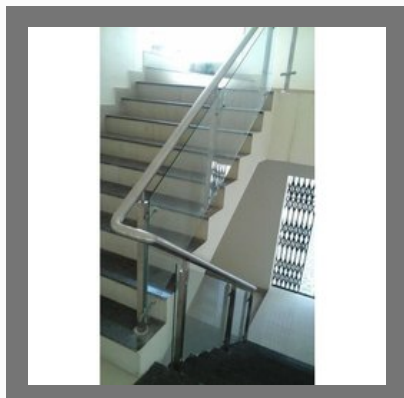
Stainless Steel Glass Stair Railing
